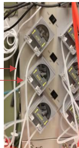
Tubing going through pump
